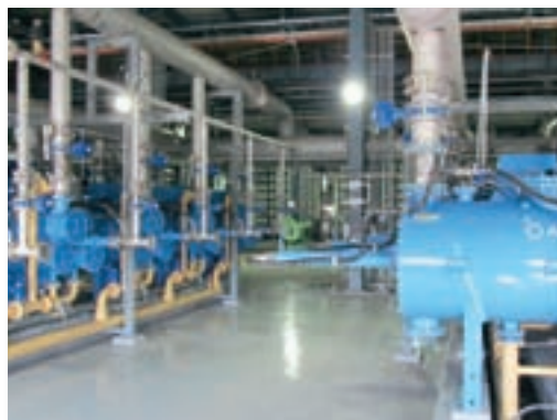
Industrial: Membrane protection for process water at a steel production plant, Korea
