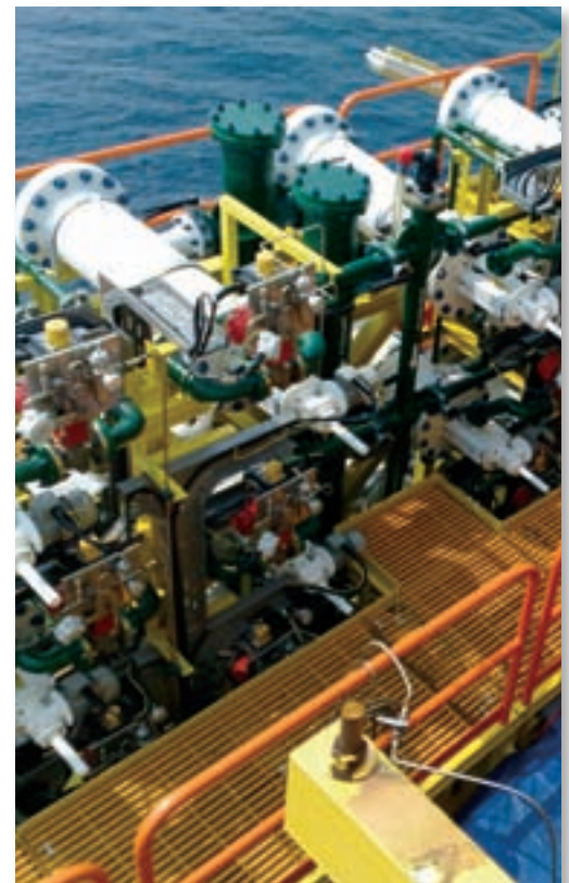
Oil & Gas: Filtration for injection water at off-shore rig, South East Asia
